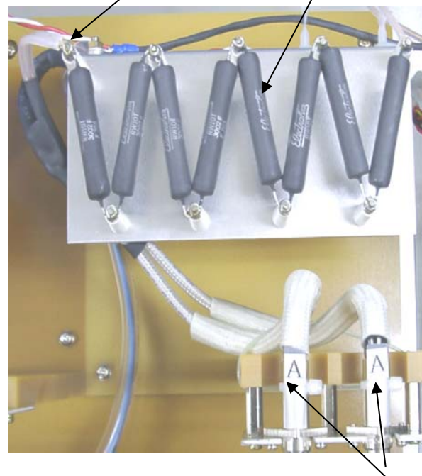
(a) Pulse forming part from a high-voltage power supply (b) It wired taking isolation voltage into consideration
